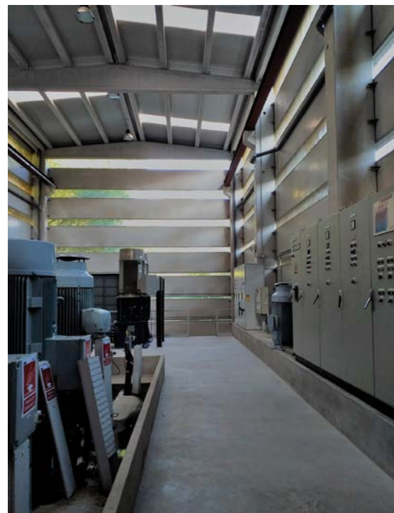
Bombeo auga potable Monte Porreiro
